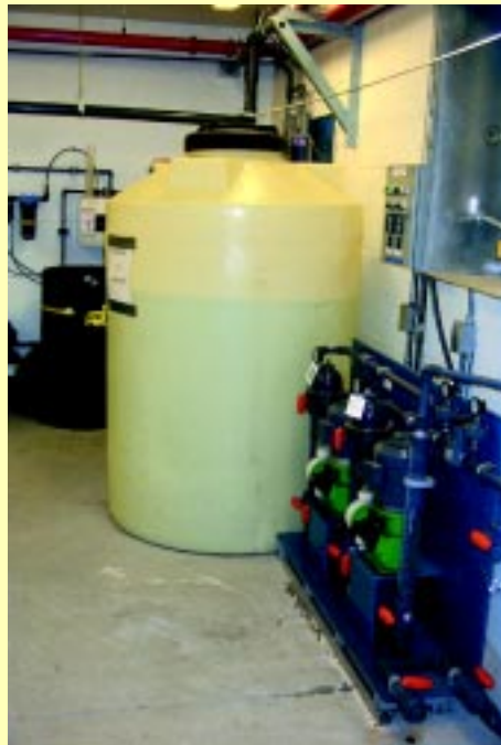
An existing sodium hypochlorite injection system, which treats water for aesthetic purposes.
