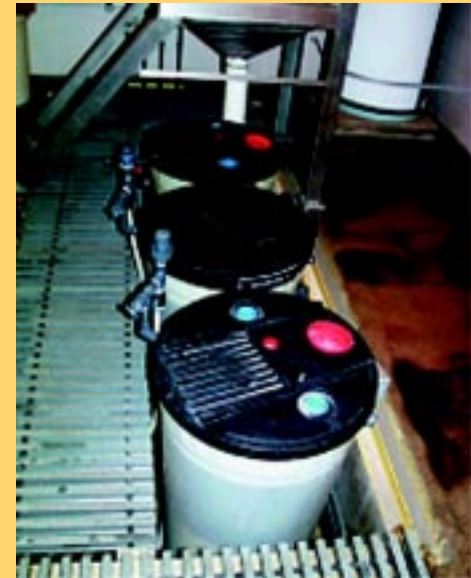
A sodium fluoride saturator tank
