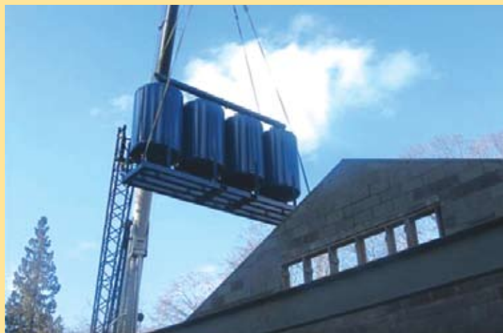
A crane was used to move the filter tanks into the facility.
